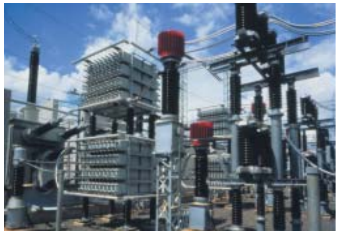
Figure 6. Commutation capacitors at Garabi
