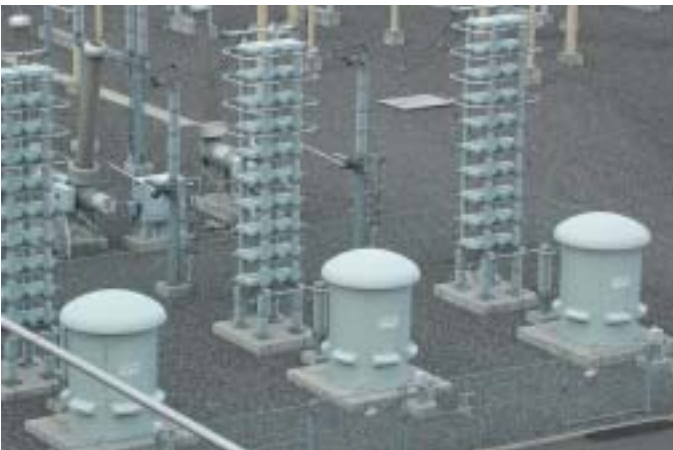
Figure 3. ConTune filter installed in the Celilo station of the Pacific Intertie HVDC transmission system
